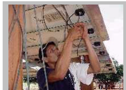
Installation and maintenance training on the 2.5 kW photovoltaic system in the rural community of Porvenir. Energy efficiency has reduced power requirements to 1.5 kW.
