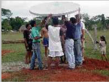
Installation training on the 1.8 meter C Band satellite dish connecting the rural community of Porvenir to the Internet through a gateway in the U.S.
