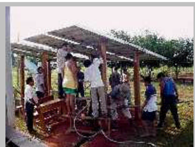
Installation training on the 2.5-kW photovoltaic system that powers 3 computers, lighting for the school, and a refrigerator for medical vaccines.
