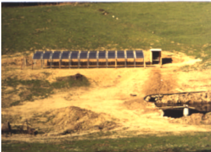
3840 Wp pump in Zigliara (Corsica)
