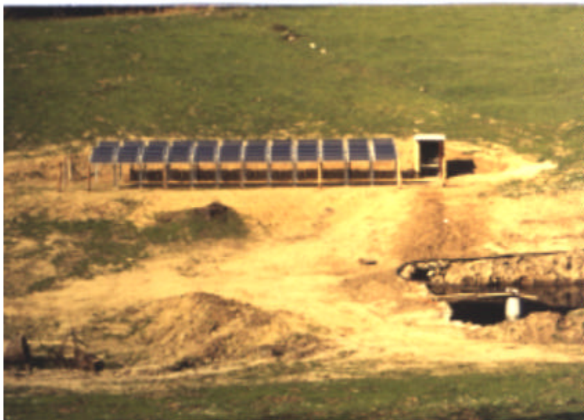
3840 Wp pump in Zigliara (Corsica)
